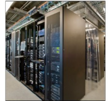
Server towers with racks
