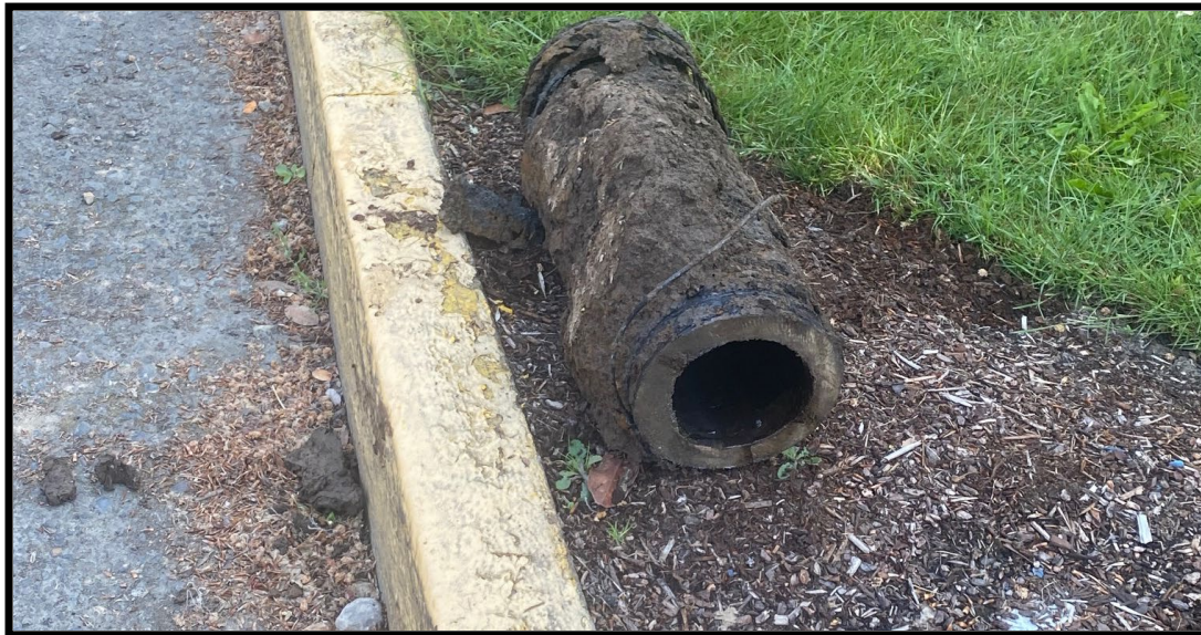
Abandoned wood pipe under Monmouth Avenue
