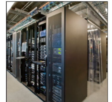
Server towers with racks
